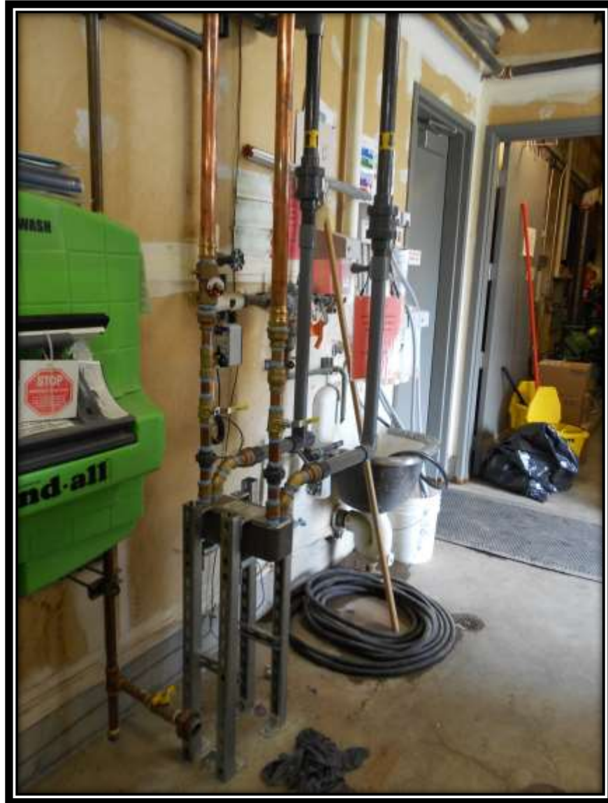
Typical heat exchanger installation replacing the existing boilers
