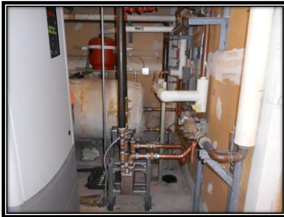
Domestic water heat exchanger
