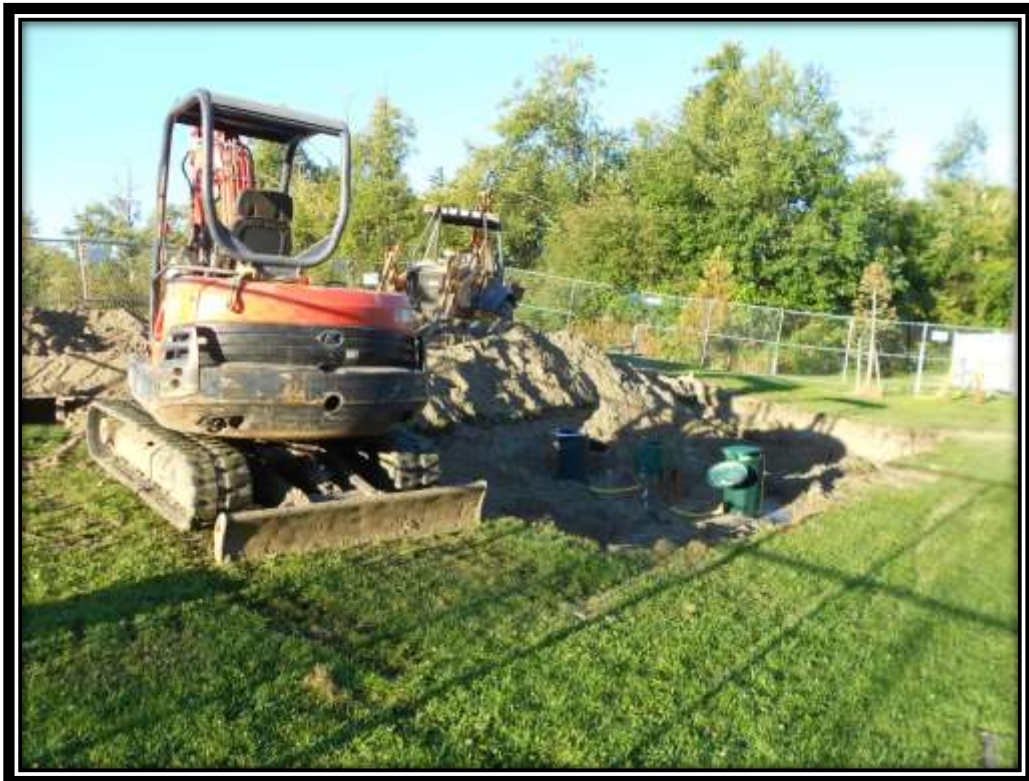
Securing the jobsite at the end of the day following earthwork activities
