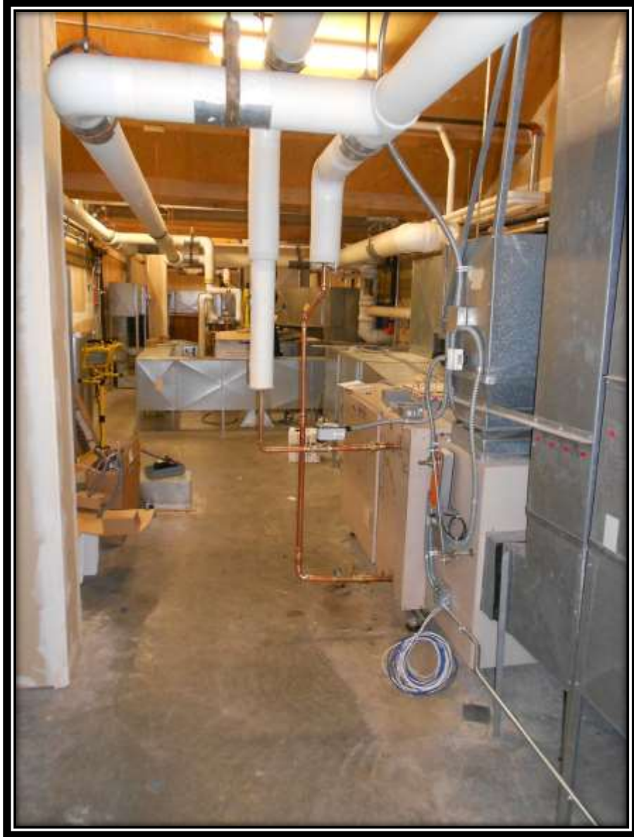
Typical attic mechanical room where new coils, motors and VFD's are installed
