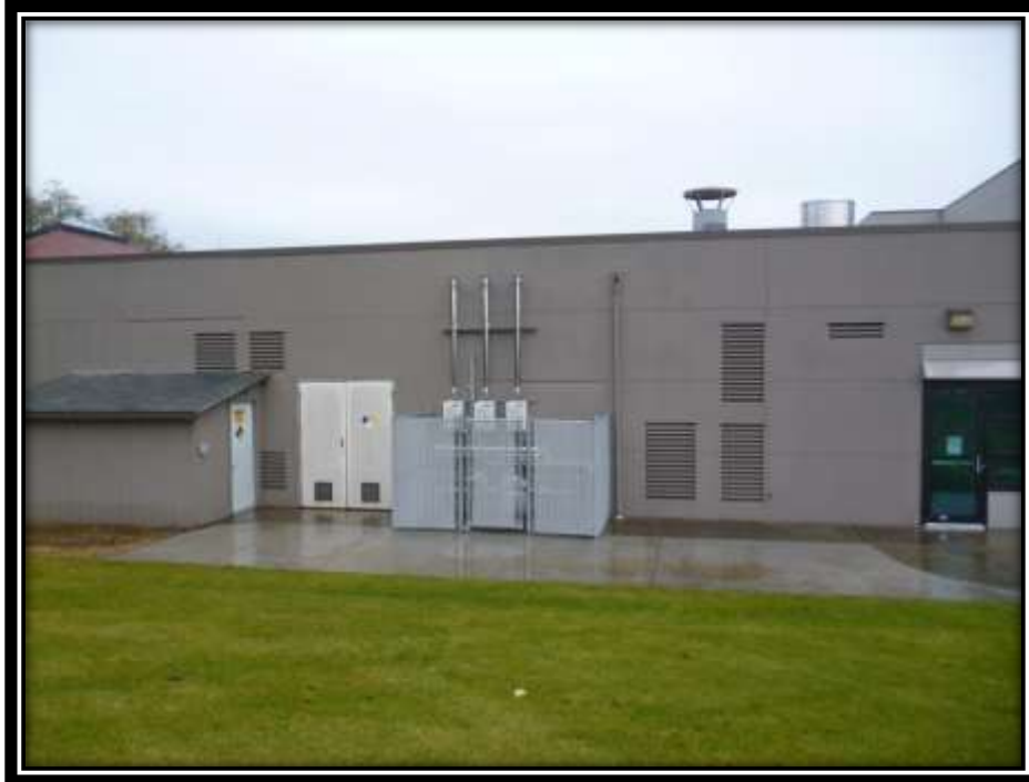
View of the mechanical room entrance and hot water heaters prior to construction
