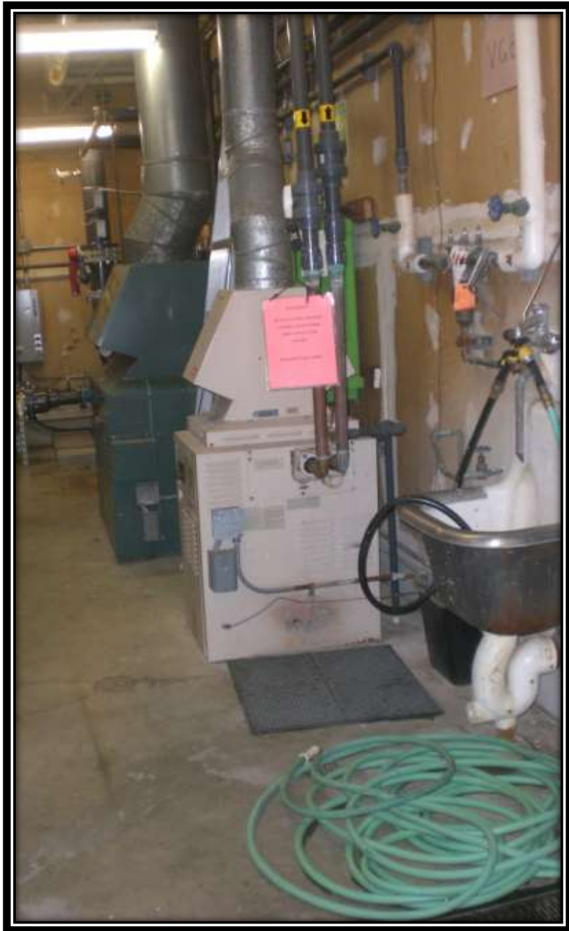
Existing Boiler #2 and #3 prior to removal and replacement
