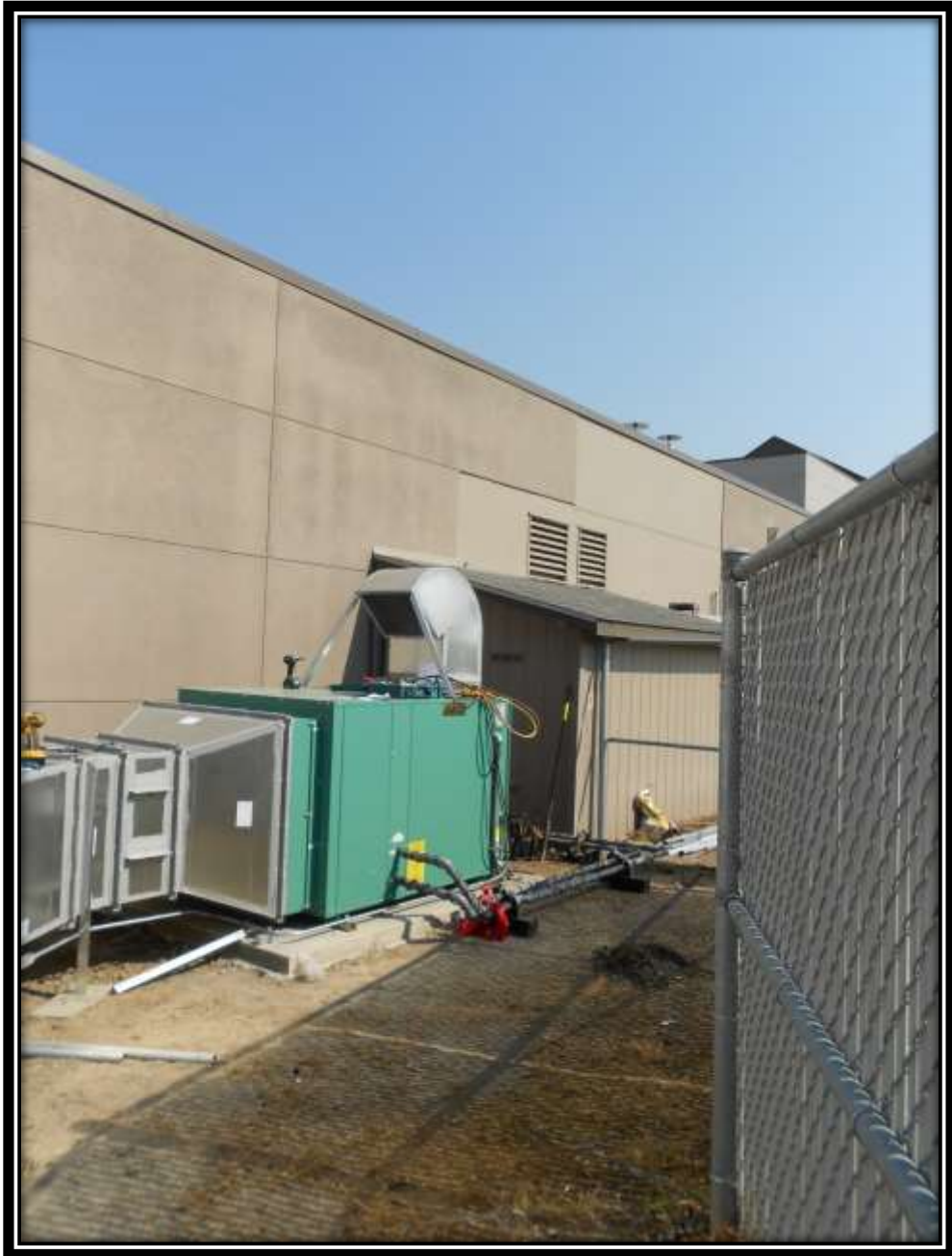
Finishing up the installation and final placement of the new outdoor unit
